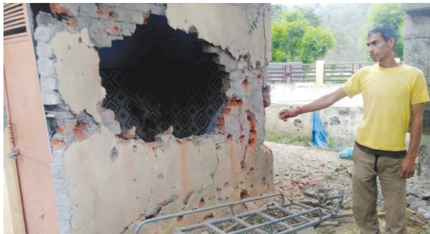
A resident living near the border points out damage caused to the wall of a government middle school by mortar shelling from Pakistan at Jhanghar area near the LoC.
