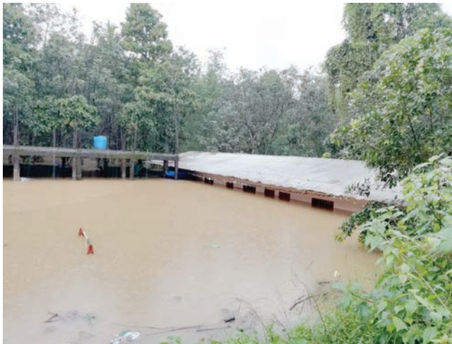
School building submerged in water during Flood Disaster
