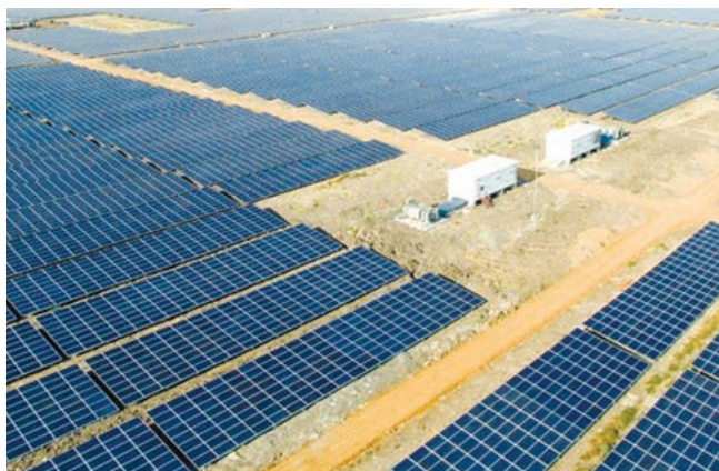
Adani Renewable Energy Park Rajasthan Limited (AREPRL) in village Nedan in Pokhran
