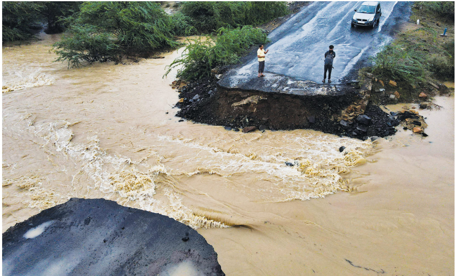
A drone view of a broken bridge after Cyclone Biparjoy made landfall along the Naliya-Bhuj highway in the western state of Gujarat, India. REUTERS
