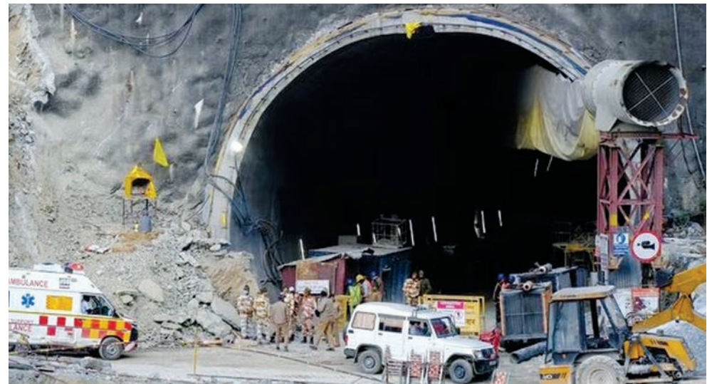
Teams at the entrance of Silkyara Tunnel during the rescue operation of 41 workers trapped inside the under-construction tunnel, in Uttarkashi district on Friday. (PTI)
