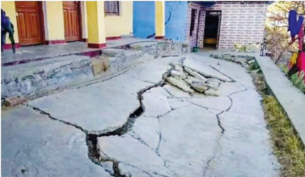
A street with major cracks due to land subsidence in Joshimath.
