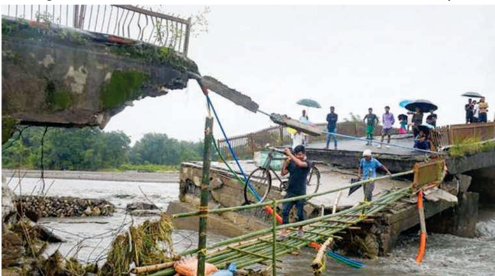
Villagers use a makeshift bamboo bridge to cross the Daranga River after the collapse of the concrete bridge due to floods at Kumrikata in Assam.
