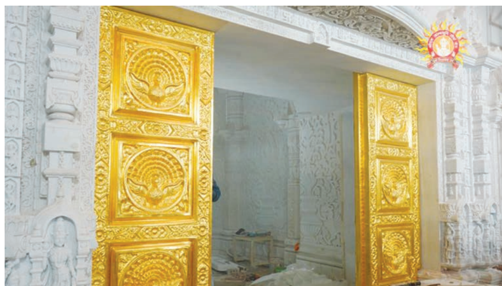
With the installation of Golden Doors in the Garbhagriha of Bhagwan Shri Ramlalla Sarkar, installation work of all golden doors on the ground floor stands completed. (Twitter/@ShriRamTeerth)
