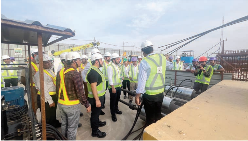
The delegation visited the casting yard and construction site of the elevated metro arranged by DMRC in New Delhi
