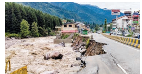
The partially washed-away Manali-Chandigarh highway is seen alongside a swollen Beas River at Manali, following a recent cloudburst in Kullu district, on August 1. PTI
