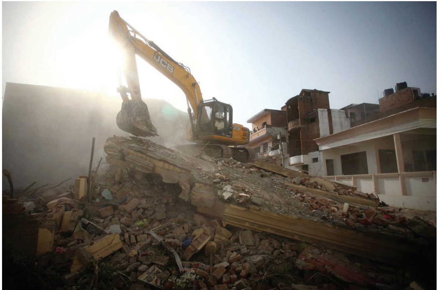
A bulldozer in Prayagraj on June 12, 2022 demolishes a house of a Muslim man that Uttar Pradesh authorities accuse of being involved in riots that erupted following comments about Prophet Mohammed by BJP members. Authorities claimed that the house was illegally built.
